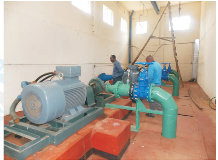
Pumping station at the water intake
